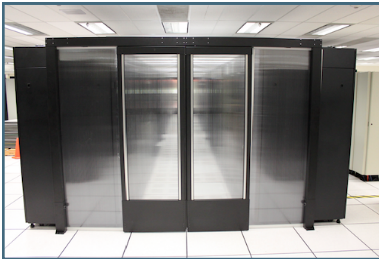
Cold Aisle Containment
