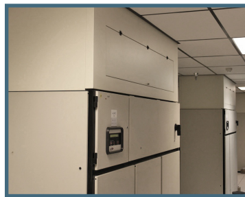
CRAC Extensions to Increase Delta-T
